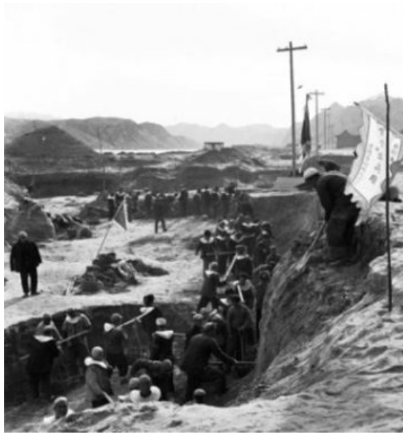
Building a cofferdam of straw and mud to divert the Yellow River at the Qingtong Gorge in Gansu, December 1958. Forced labour on water conservancy schemes all over the country claimed the lives of hundreds of thousands of exhausted villagers already weakened by hunger.
